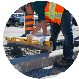
Pot Hole and Curb Pe-Maintenance
